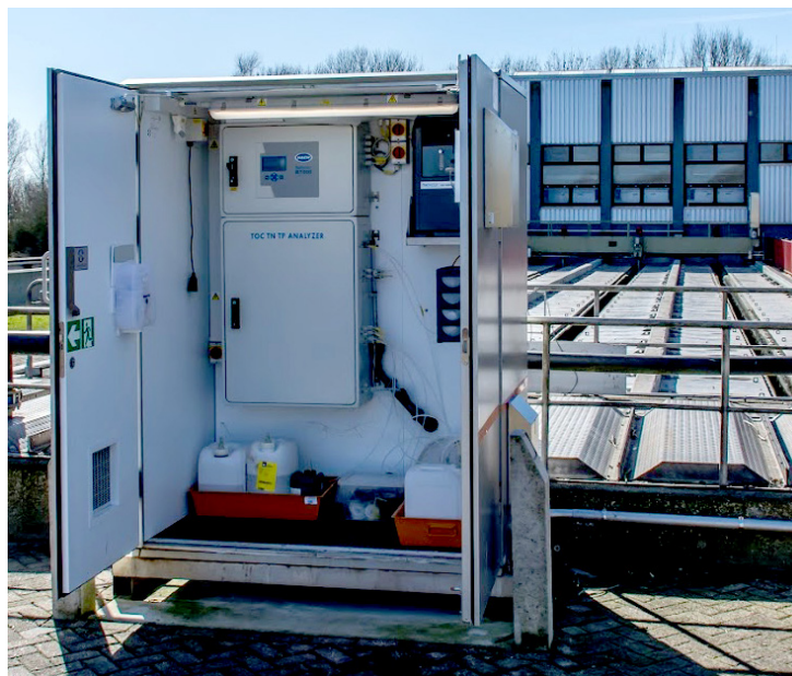
Biotector unit at the Oijen WWTP
